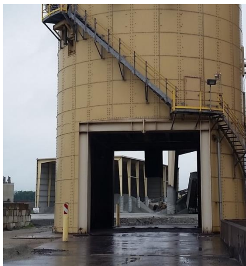
Figure 3-5: U4 Fly Ash Loading Operation
