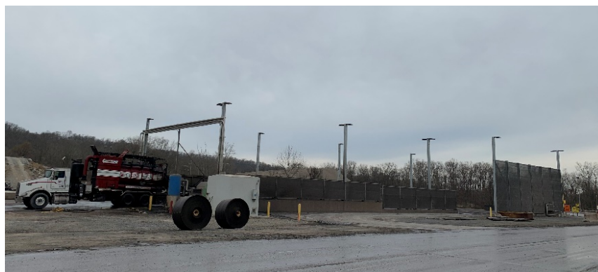
Figure 3-12: Vacuum Truck Ash Handling Station Loading Operation
