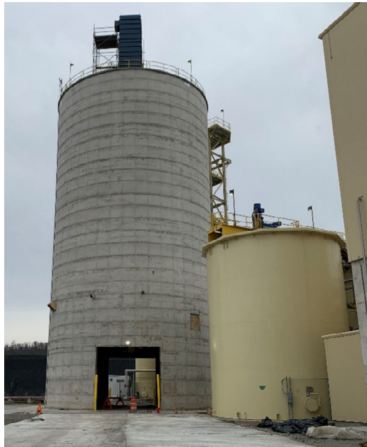
Figure 3-11: New U1/U2 Fly Ash Silo Loading Operation
