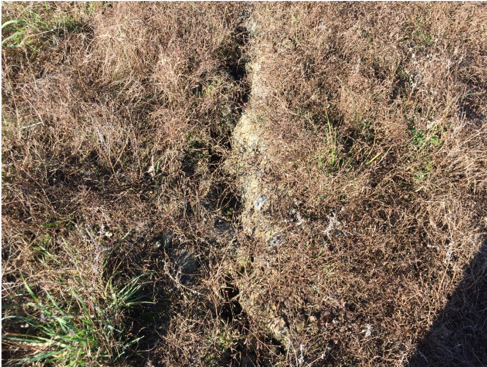
Photograph Number : IMG-7485 Description: Outside the landfill limits - Evidence of slough above Pond 1, north slope
