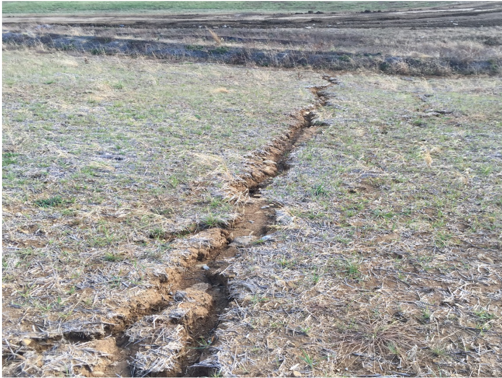
Photograph Number: IMG-7543 Description: Final cover erosion, west and south slopes
