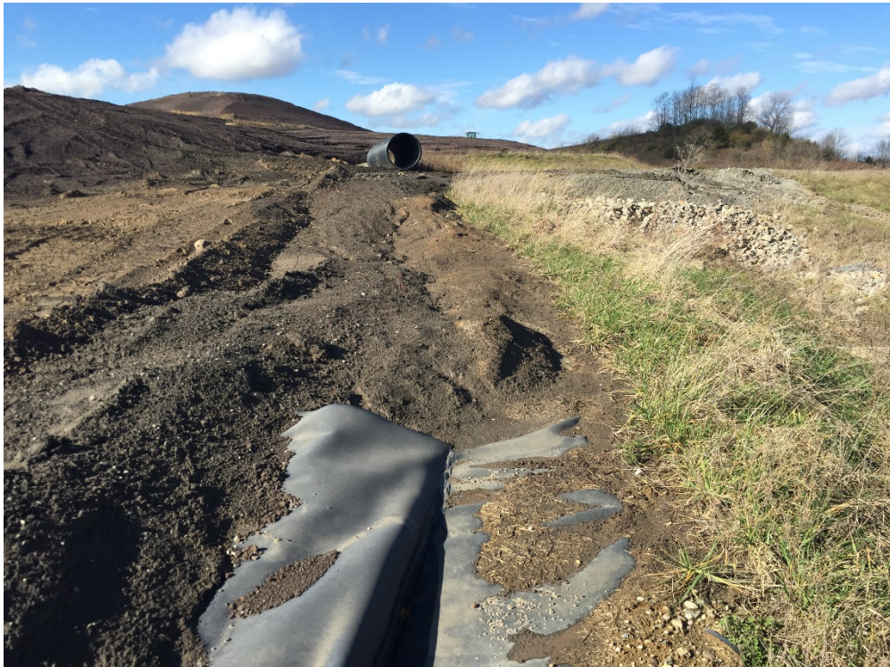
Photograph Number: IMG-7523 Description: CCR outside the north waste limits of Area C, Phase 2
