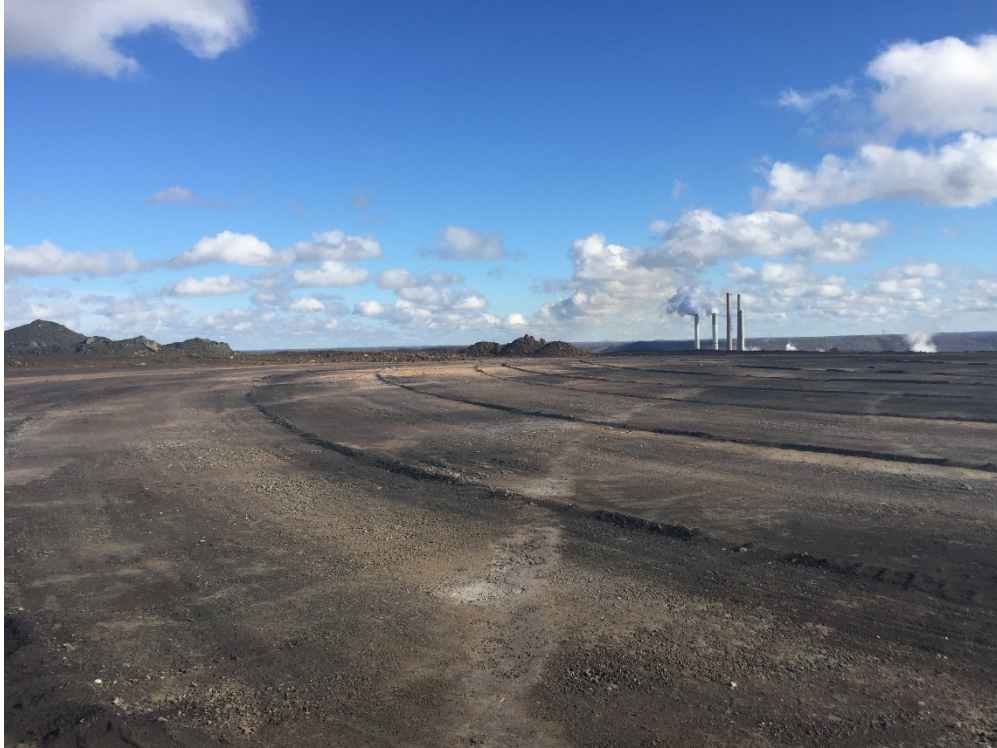
Photograph Number: IMG-7514 Description: Area C, Phase 1 working face/fill area, looking north
