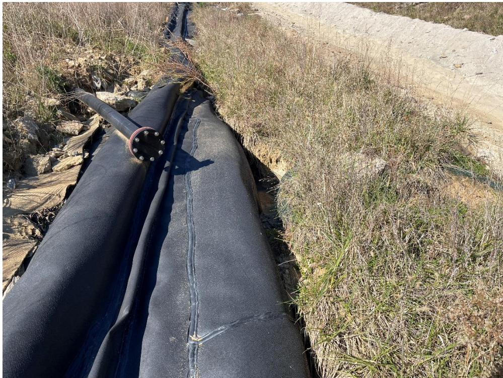
Photograph Number: IMG-2566 Description: NE Area C phase 4 – Anchor Trench erosion
