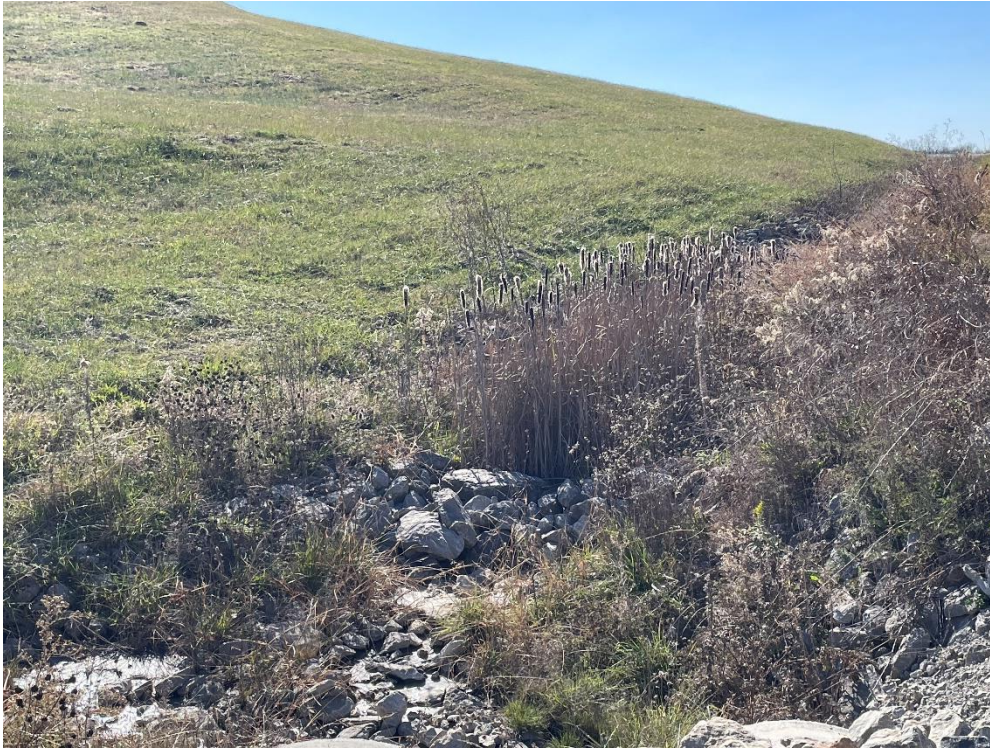
Photograph Number: IMG-2541 Description: West final cap, NW ditch – Woody vegetation growth
