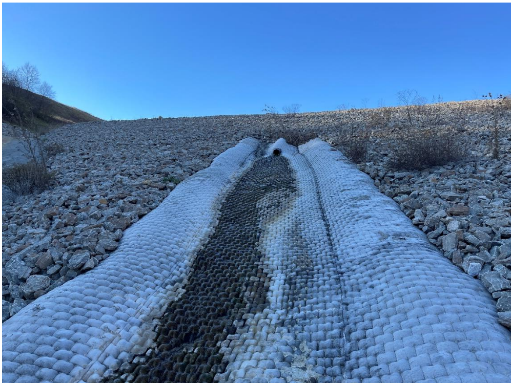
Photograph Number: IMG-2620 Description: Leachate Discharge to Pond 1
