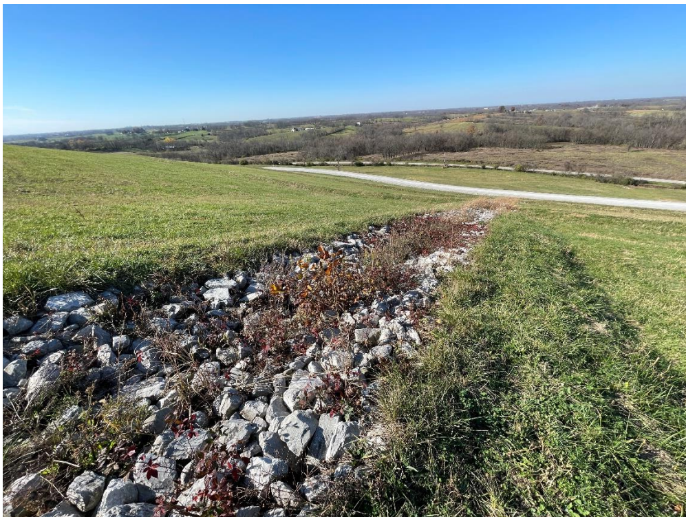
Photograph Number: IMG-2494 Description: West Final Cap, north downdrain – Woody vegetation growth
