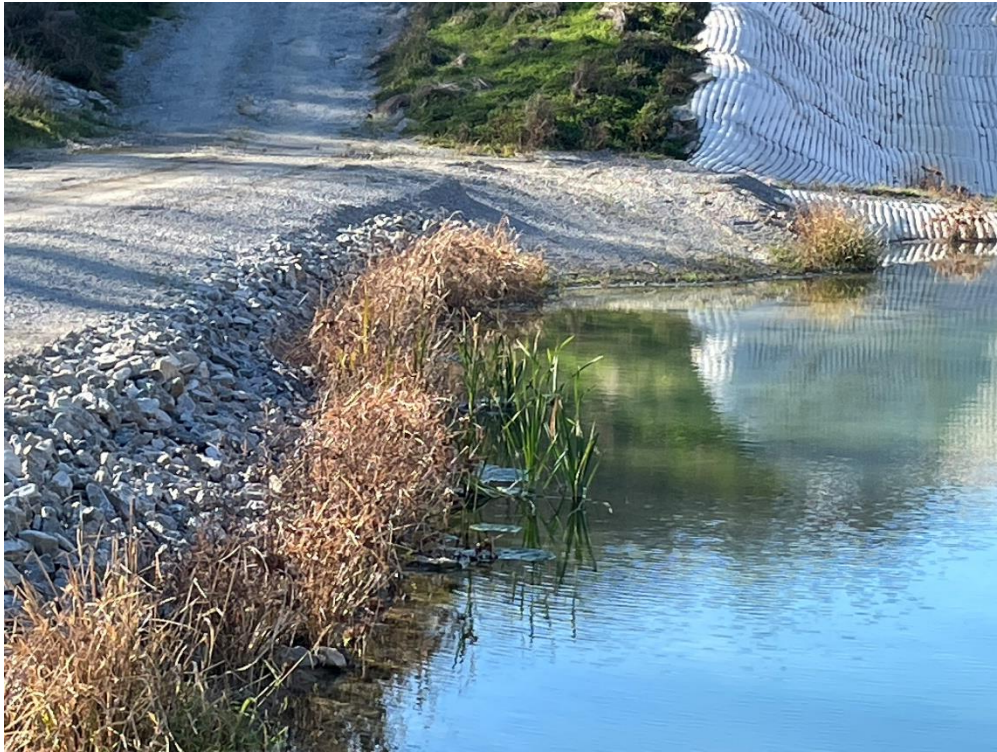
Photograph Number: IMG-2601 Description: Pond 2A – Woody vegetation growth
