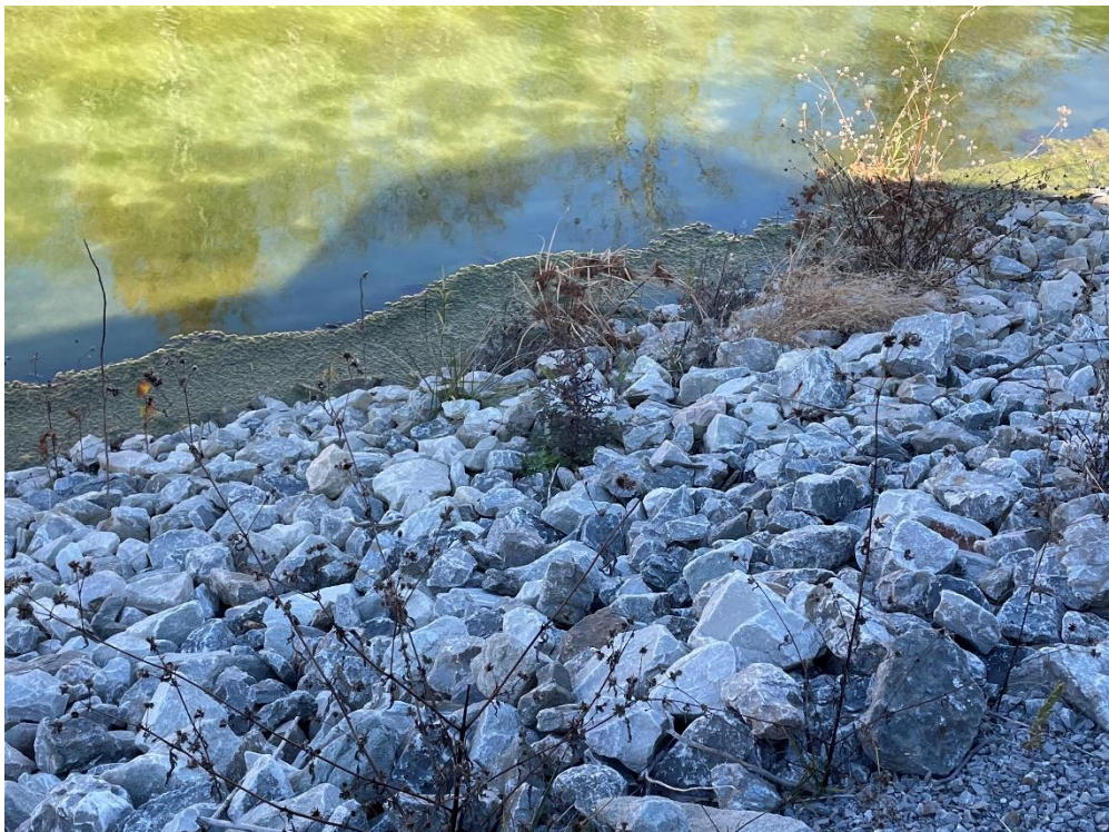
Photograph Number: IMG-2604 Description: Pond 2A – Woody vegetation growth
